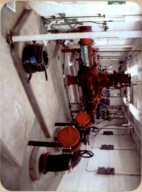
Cooling Tower Recirc. Pumps
